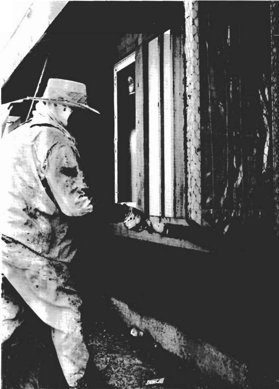
Workmen are blowing the first coat of stucco on one of the specially built MED homes. Beneath the stucco is 8 mil plastic wrap — rather than standard tar paper — to help seal the homes from outside air. Vertical shading wings reduce the amount of sunlight striking the double-pane windows.
